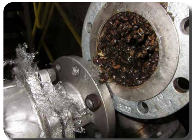
Six-inch process water intake pipe clogged with zebra mussels. Photo taken at an industrial facility in Michigan.
